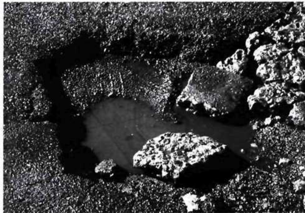
The poor condition of SA's national, provincial and municipal roads contribute to 20% of all road deaths
