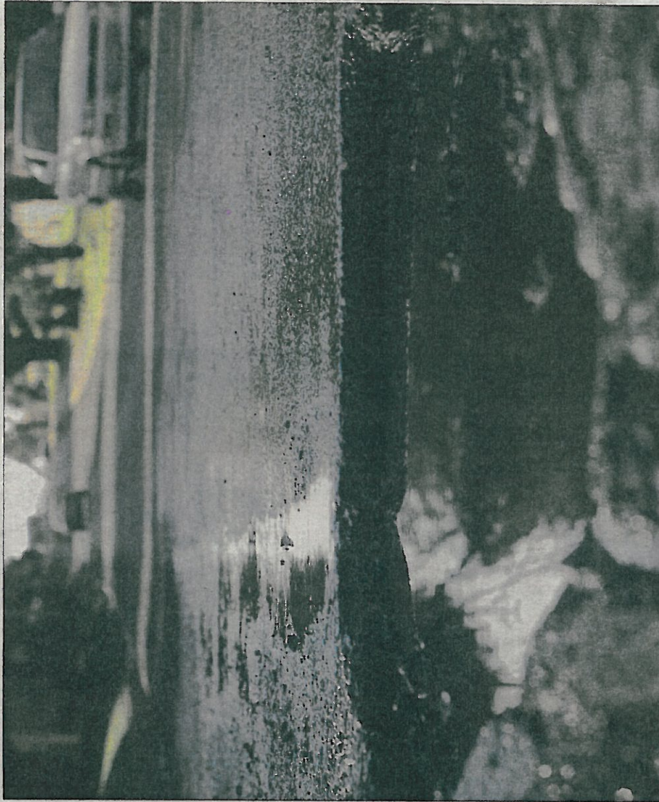
SINK OR SWIM: Dangerous potholes, like this one, are nice for ducks to take a dip in, but they cause a lot of damage to cars and people and are expensive to fix – simply because there is no proper road maintenance taking place.
